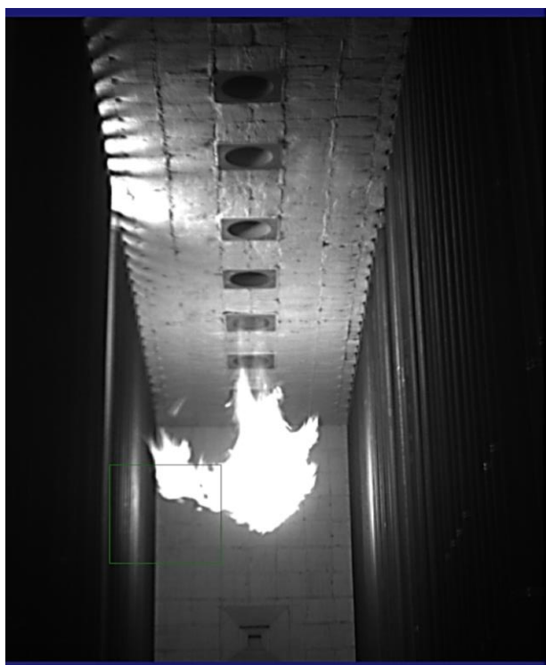
Figure 3. First SMR burner light off
